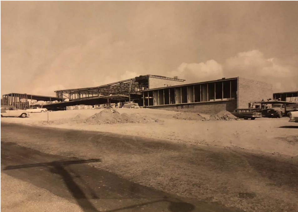
Figure 8. Construction, c. 1959. Camera facing northeast from Ridge Road. Notice the curvature of roofline. Compare to Figure 4 and Photographs 7-8.
