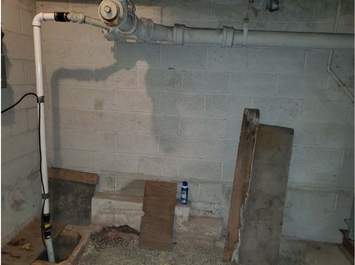
Photo from Broken Sump pump pit in Basement near Front Entrance
