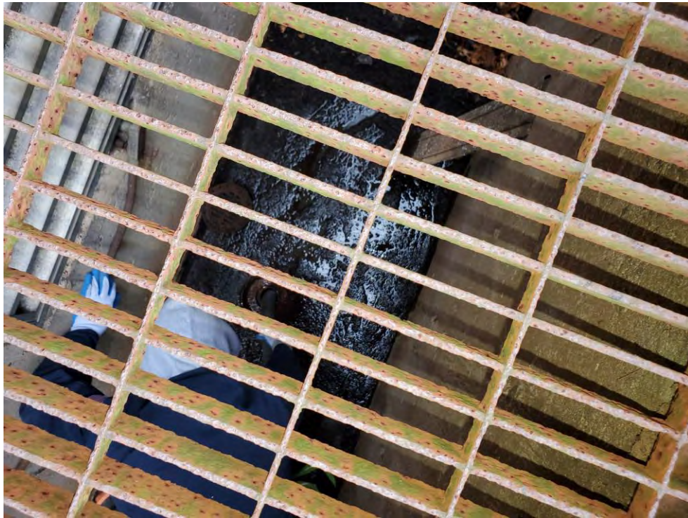
Photo from Drain Inlet #1 Before Clearing
